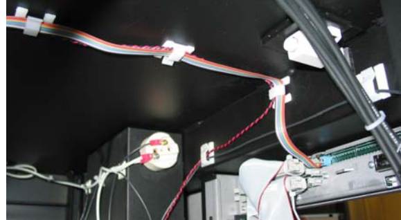
Cable routing on the CEM3 side
