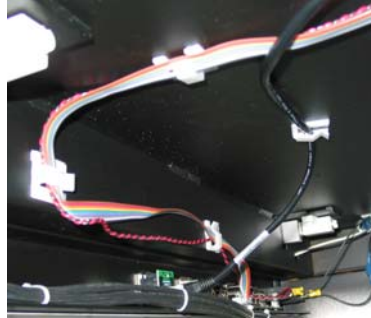
Cable routing on the input panel side
